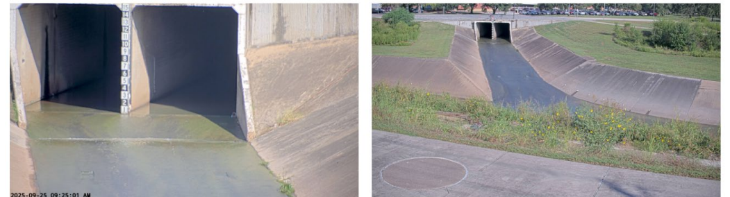
Bayou cameras provide vital water levels and visual confirmation during a flood event. The Harris Gully Gage was selected as the critical point to view gage activity for the Rice/TMC system. Gully levels are automatically communicated to TMC.
